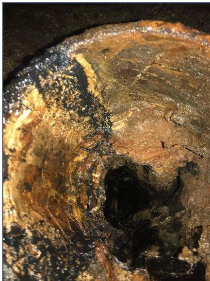
BFP Drain Line Plugged
